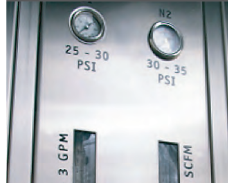
Facility Panel Controls All Pressures and Flows
